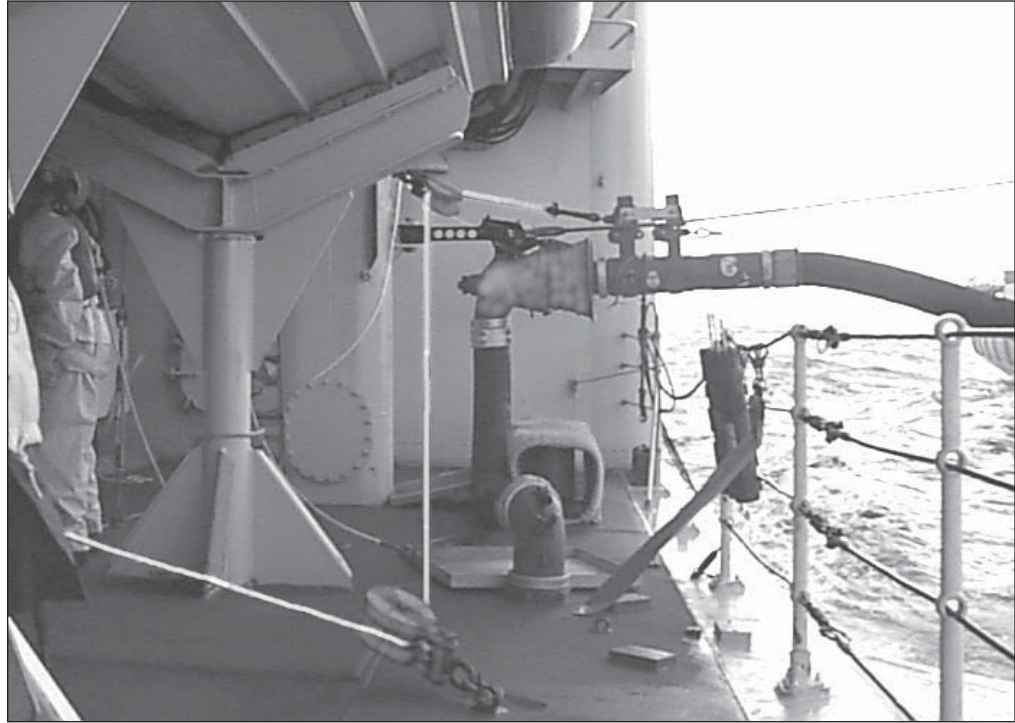
Figure 9.21-10 - Liquid RAS Station 4
